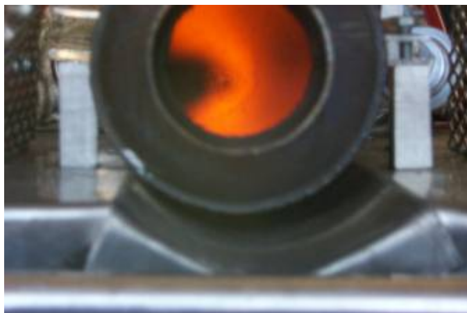
Figure 21: Black Local Section of Failed Catalyst Wash Coat
