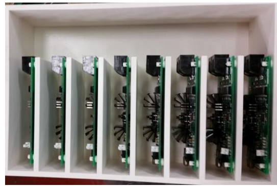
Figure 17: BMS rack enclosed in battery box
