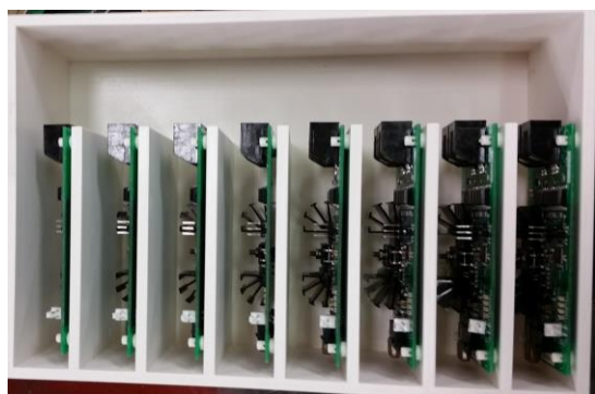
Figure 7: BMS rack enclosed in battery box
