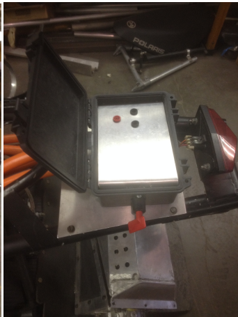
Figure 10. Measuring Point access
